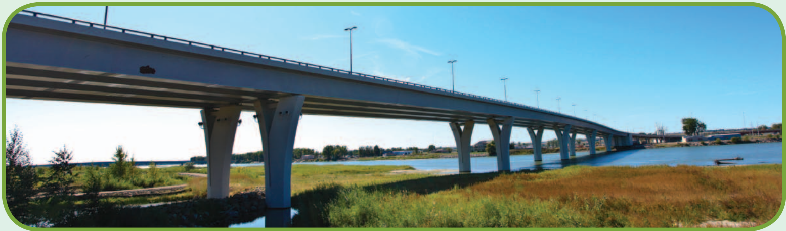
Coal ash was used as an additive in the concrete used to build the new Memorial Bridge across the Missouri River in Bismarck, ND.
