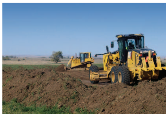
Construction crews started moving dirt on Oct. 5 for the cooperative's latest wind project in south-central South Dakota.
