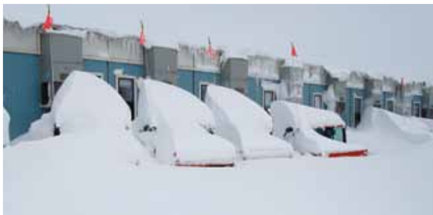
The same storm that hampered the flood response in North Dakota in late March first hit Gillette, WY, on March 23. Heavy snow accumulation and near-zero visibilities stopped construction on the Dry Fork Station for about a day. The blizzard buried four Kubota tractors on site, shown here in a photo taken March 24.
