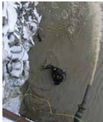
A diver prepares to set a diesel-powered submersible pump near the intake of the Leland Olds Station. The pump provided water to the fire protection system while the power plant was off line.
