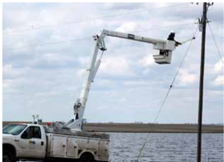
A Dakota Valley Electric lineman braves the flood waters to repair a distribution line.
