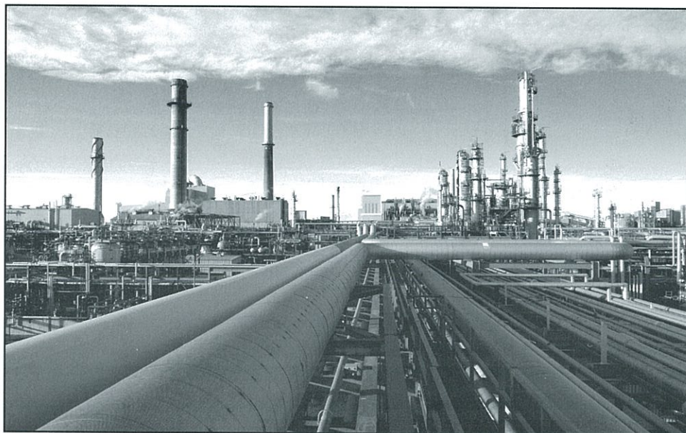
Pipes carry many fuels and liquids throughout the Great Plains Synfuels Plant in Beulah, ND.
